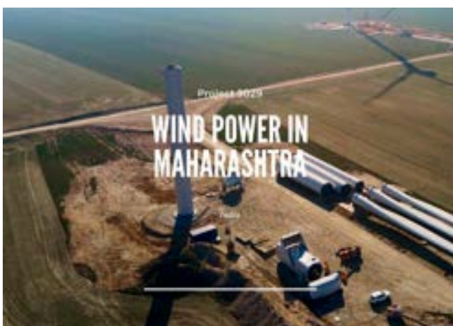
Project 3029: Wind Power in Maharashtra
